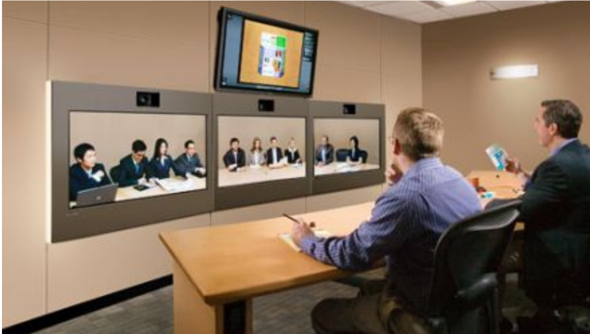
Figure 6 – A representative installation of the HP Halo system illustrating a typical meeting configuration.
